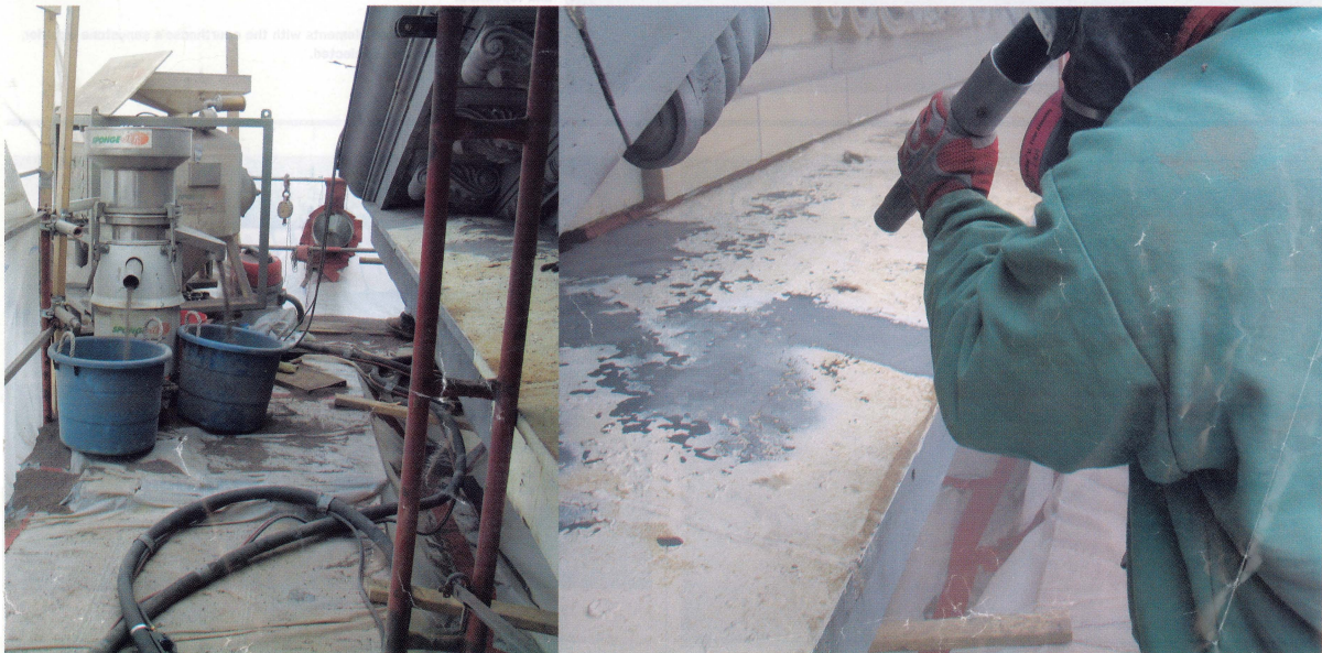
The Sponge-Jet blasting system was located on the same level as the work being done, allowing blasting and recycling to be carried out within feet of the blaster.
